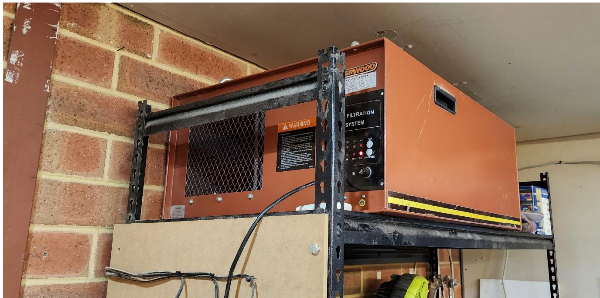
Machine room air filter
